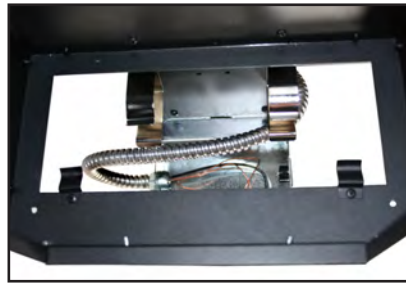
8. Feed Conduit through top access and connect conduit to J-Box through side access Panel
